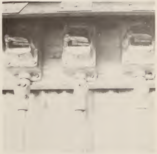
SHELF PROTECTS SWITCHES
